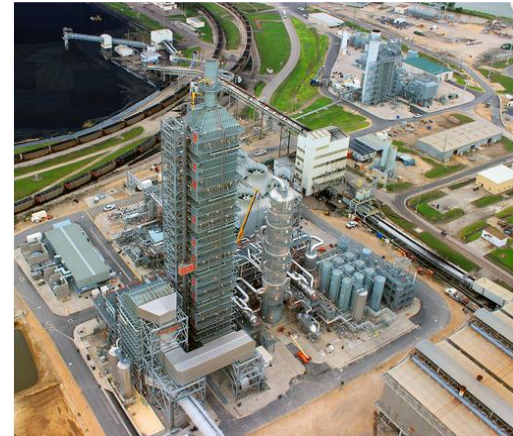
Carbon capture facility. Absorber Tower in the foreground. Regenerator Tower next to it . Co-generation system at the top right
