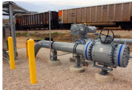
The CO 2 is used for EOR. Sent through this pipeline inlet at ~ 130 bar
